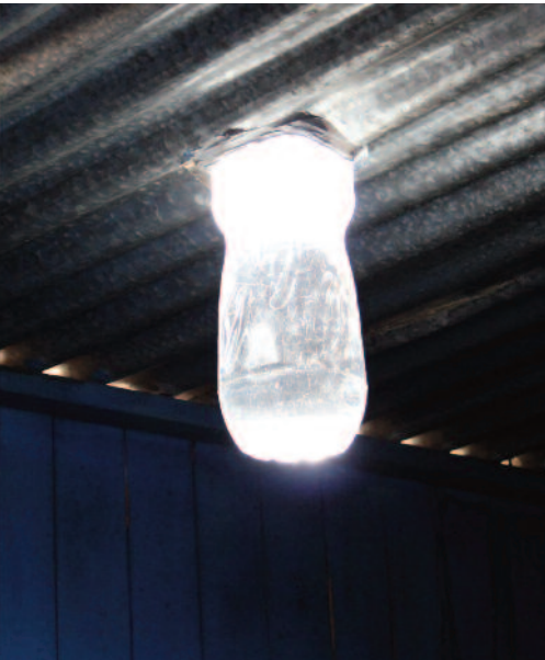
At the volunteer project in Peru we have showed youth in the slums how to install solar light bulbs and become entrepreneurs on the field.
